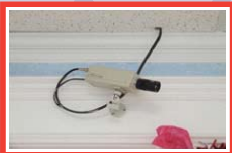
Interior Camera Installation
